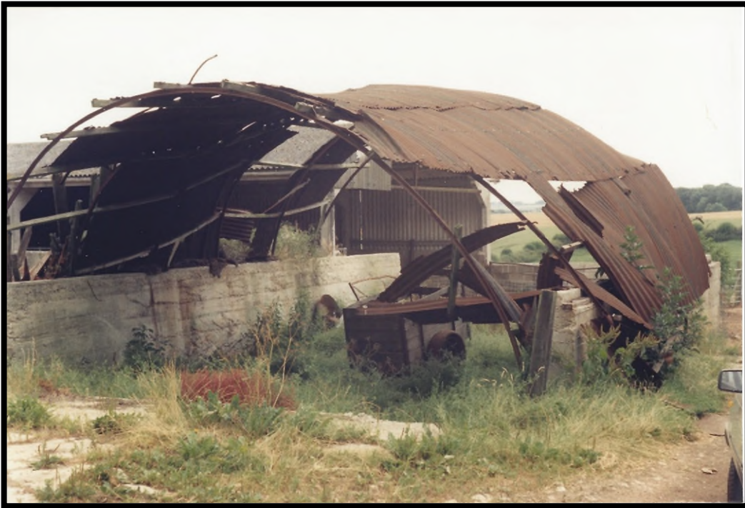
Figure 6: Derelict corrugated barn at Lower Farm, Upper Milton, before reclamation of the site in the 1980s.
