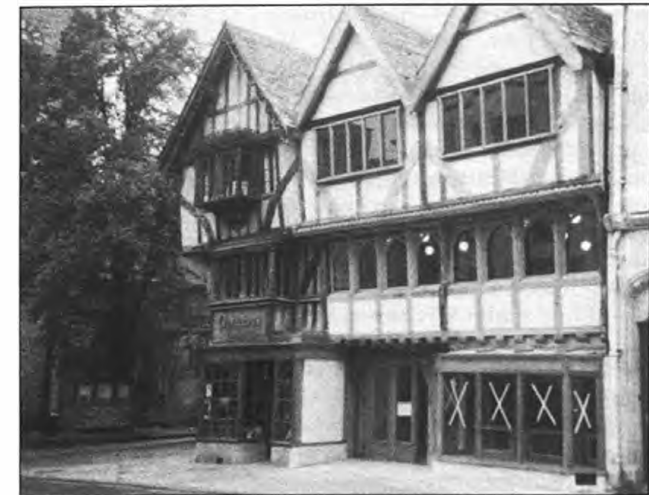
Nos. 26 and 27 Cornmarket, Oxford, formerly the premises of Zacharias & Co, gentlemen's tailors, and all that remained of a fourteenth-century inn. Seen here after restoration by Alfred Groves and Sons.
